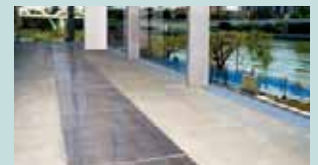
HVAC grates satisfy form and function - Page 2
