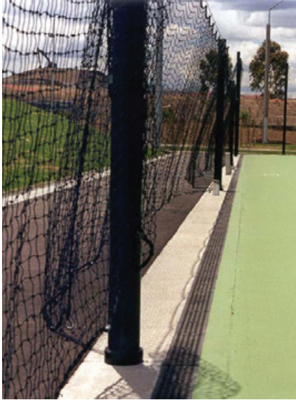
Rosette gratings in K100S channel around perimeter of practice courts
