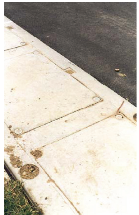
ACO brass edged access covers filled with concrete located alongside main driveway, note brass identification plate for pit contents between cover and bitumen driveway
