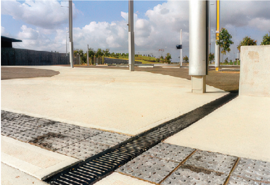
The main car park area to the west of the site is on a slight slope. Runs of S170 drain surface water away from the bus loading areas
