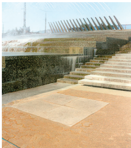
An ACO recessed galvanised steel multipart cover over the pumping system for the Northern water feature
