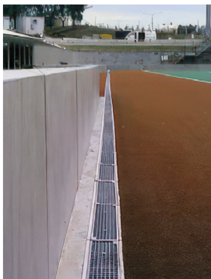
The ACO Drain N100 and Mesh grates in front of the main stand - note the wavy installation !
