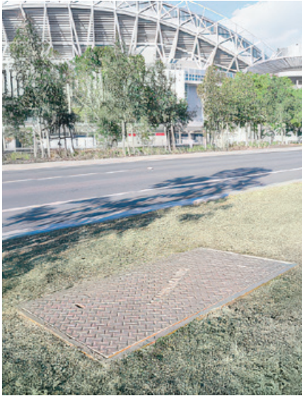
Type 95 Polymer concrete pit used for irrigation pits outside Stadium Australia
