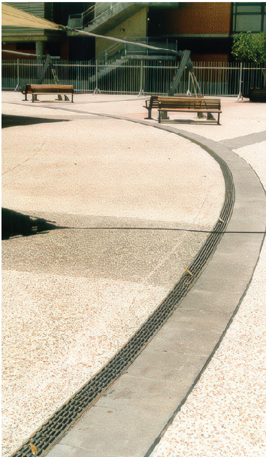
K100S drainage channel with ductile iron Intercept grate within RAS precinct
