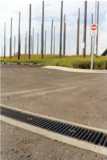
ACO Drain K200S with slotted ductile iron grates across car park entrances
