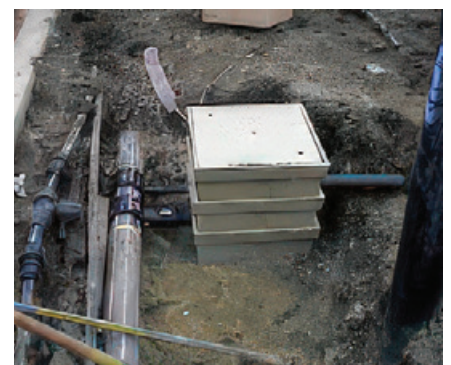
Polymer concrete pits with steel chequer plate covers outside Homebush Entertainment Centre
