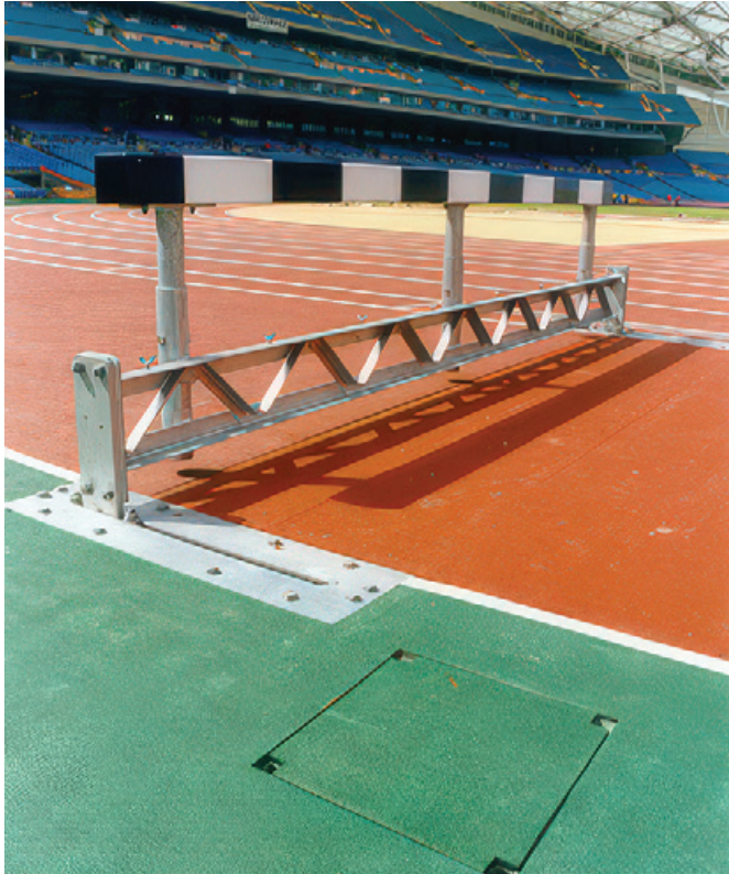
An ACO access cover used to cover the valves for the steeplechase pit
