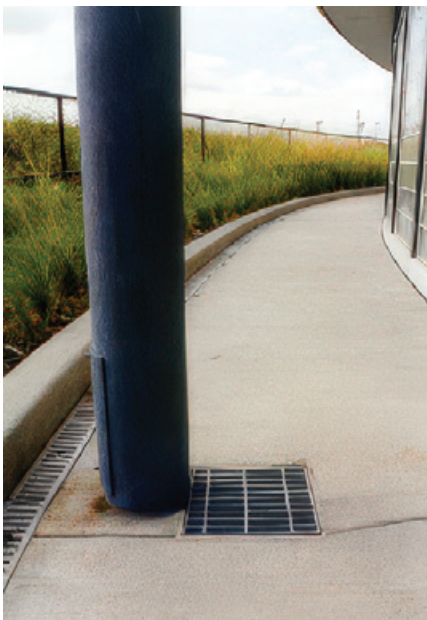
Around the rear of the main car park ticket office and amenities are runs of ACO Drain K100S and Slotted galvanised steel grate and polymer concrete sumps with galvanised grates
