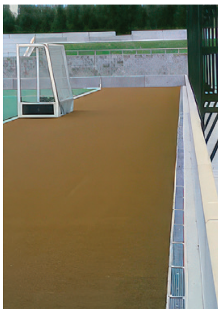
The run of N100 and Mesh grate around the perimeter wall
